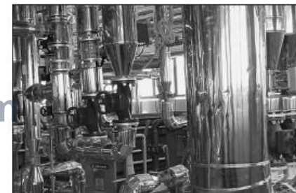
Industrial applications Courtesy UMDE Engineering, Contracting, and Trading. Used by permission.
