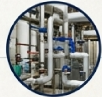
Piping and plumbing systems Photo by John M. Cimbala.
