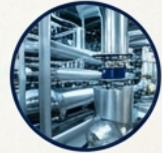
Industrial applications Courtesy UMDE Engineering, Contracting, and Trading. Used by permission.
